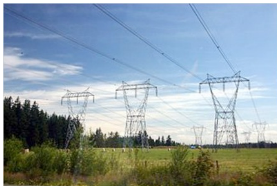
Three-phase electric power transmission lines
